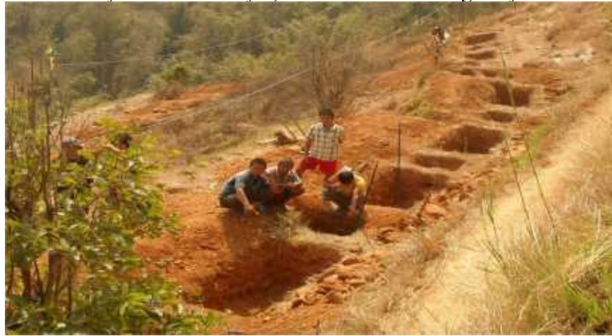
Figure 3: Artificial recharge structures comprising of rows of rectangular staggered contour trenches (2m x 0.8m x 0.6m) with square pits in between for mandarine orange horticulture plantations under construction in privately owned sloping lands in the recharge zone of Malagiri Dhara, Lungchok Kamarey Gram Panchayat, South Sikkim during May 2010
